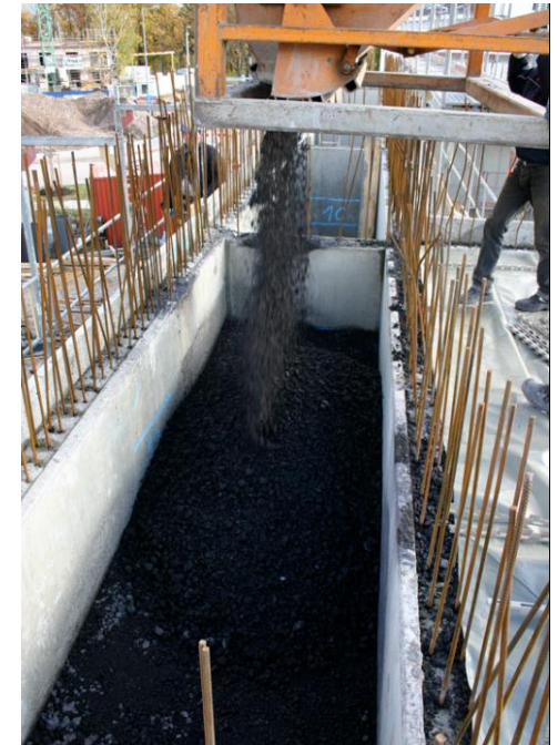
CALA radiation shielding solution, Munich. Cast in situ solution
